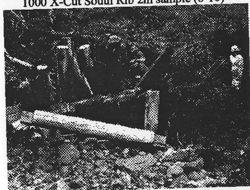
Partially Collapsed 1100 Portal
