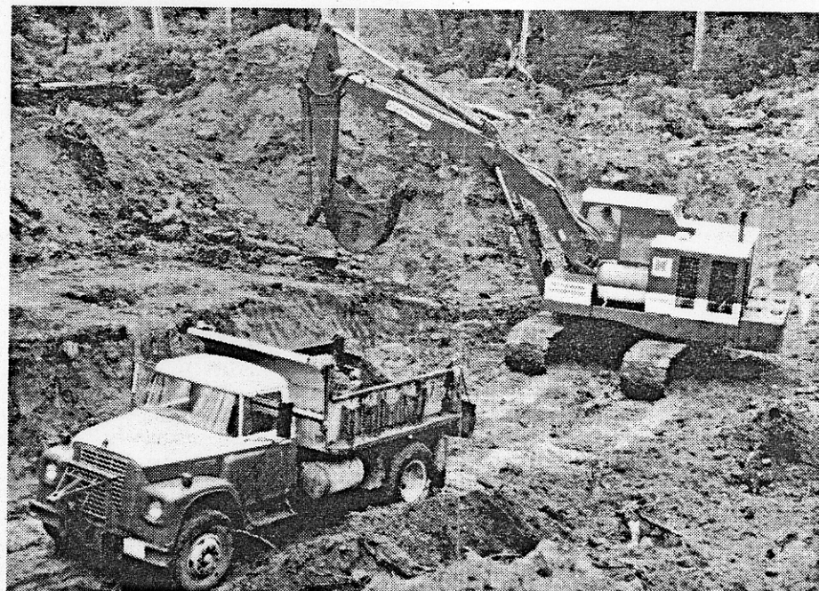
Kettle River's large excavator and dump truck, used in digging through the 10 feet of glacial sand covering the compacted river gravels on the company's Tulameen River property in the Princeton-Tulameen area of southern British Columbia. This channel sampled well in coarse gold and platinum, and permits have been secured for a testing program.
