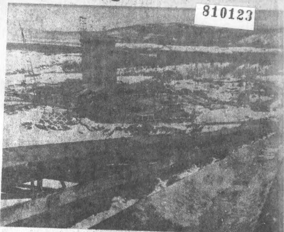
WORKMEN at Portage Mountain dam project on Peace River are now preparing the 15,000-foot conveyor system for startup on final year's fill operations. About 12 million cubic yards of material remain to be placed. The conveyor belt is
