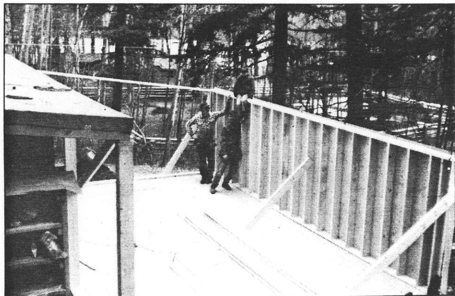
X-Cal crew at work on the addition to the company's field office in the Bridge River/Bralorne area of British Columbia. Construction is expected to be completed this month.
