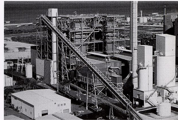
AES Hawaii uses state-of-the-art clean coal technology based on a Circulating Fluidized Bed (CFB) boiler that makes the plant one of the cleanest in the world.
