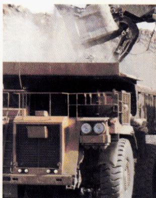
Turnagain property has excellent infrastructure and is amenable to low cost open-pit mining
