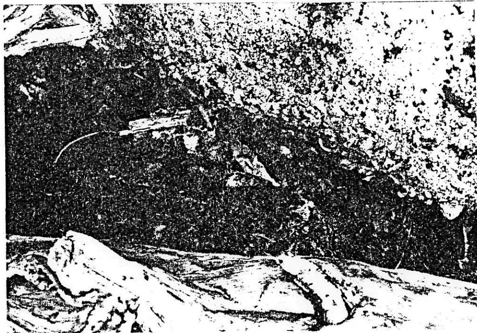
Concrete deterioration at the interface of the ogee spillway crest at the right abutment. Note: deterioration extends 8-10" into the concrete exposing reinforcing steel.
