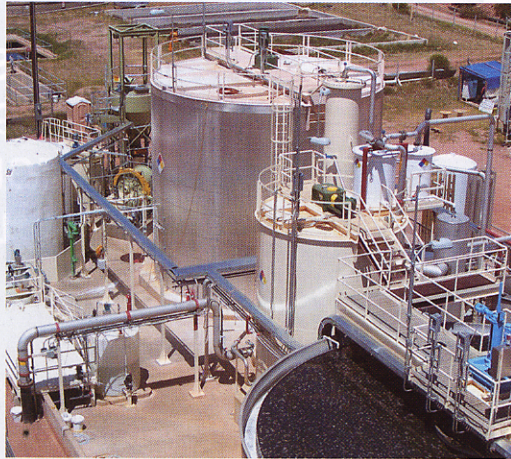
The BioteQ plant at the Phelps Dodge Bisbee Copper Mine in Arizona. Photo courtesy BioteQ Environmental Technologies Inc.
