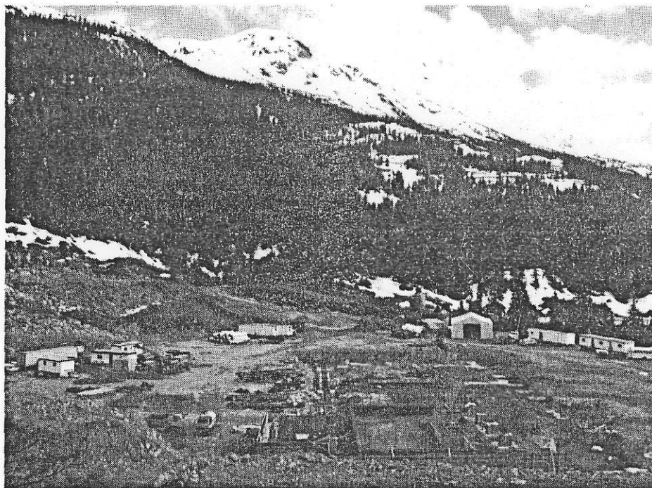
The Premier Gold millsite under construction, looking south toward the Silbak Pit.
