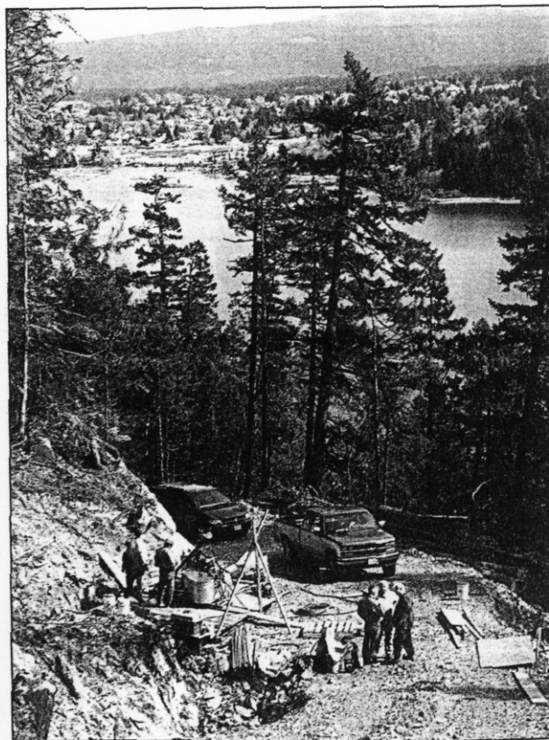
Drilling the Dauntless property. The Town of Port Alberni can be seen in the distance. Photo by Ellsworth Dickson.
