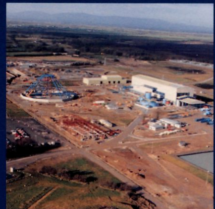
The new Lisheen zinc mine in Ireland, which commenced production build up in October 1999
