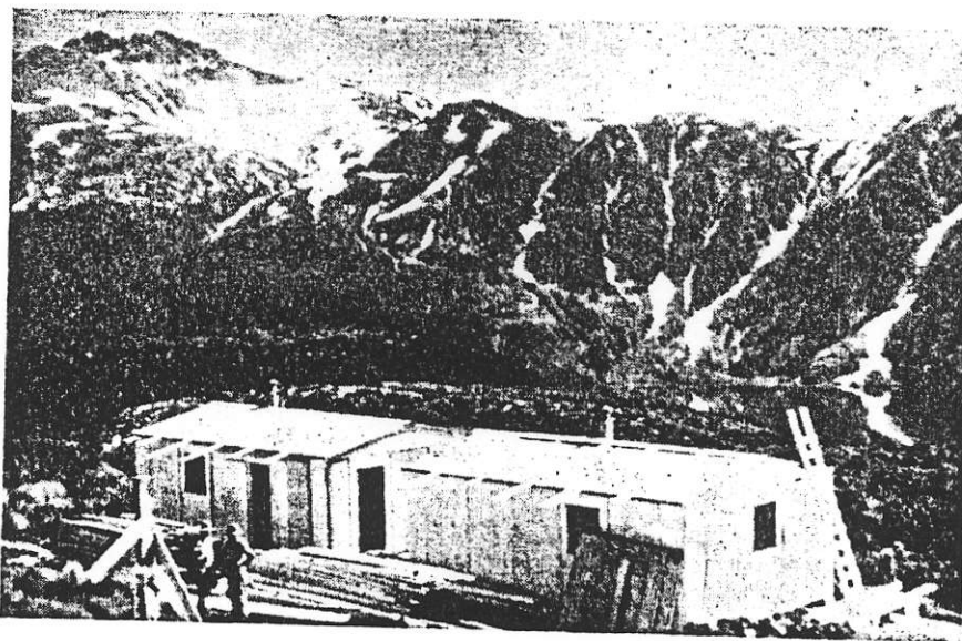
The Deer Horn mine camp under construction. Underground operations will be carried on all winter.
