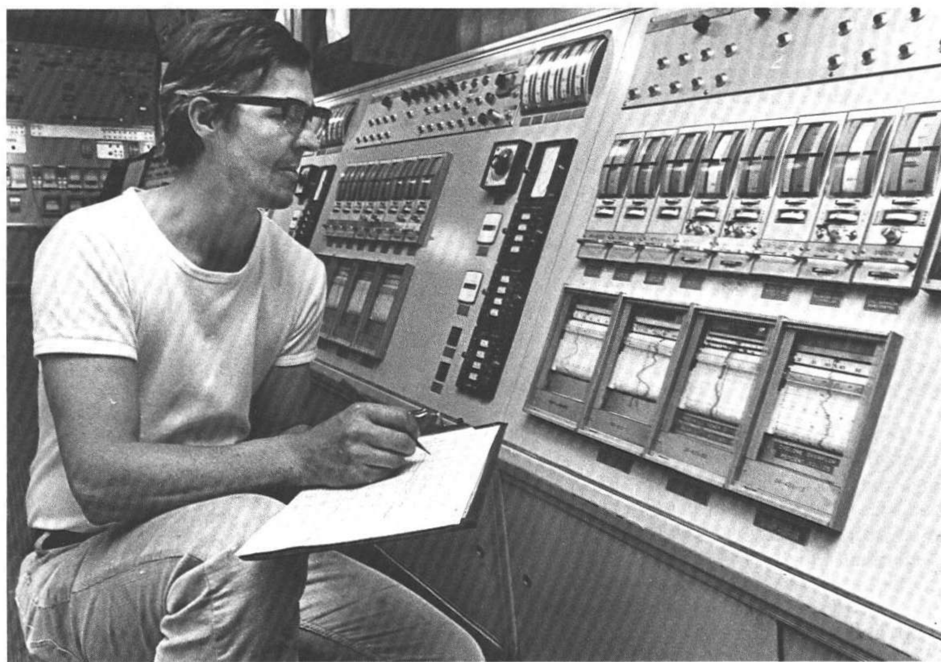
Operators in the mill's central control room (CPI) monitor the entire milling operation using closed-circuit TV cameras and other electronic devices.
