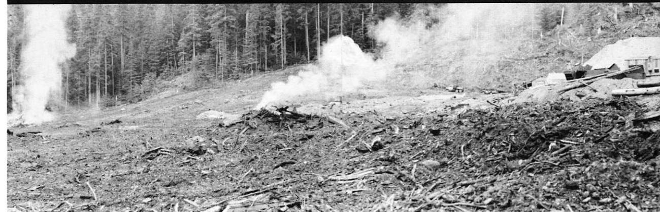
Clearing in progress on the Lynx Site for the Western Mill and related surface installations.
