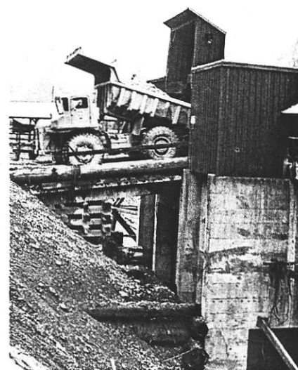
Truck dumping ore from Myra mine into storage and crushing area to begin the milling process.
