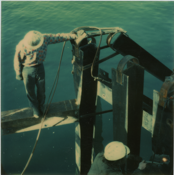
DOLPHIN DAMAGE (2nd From S) EASTER WEEK-END 1975
