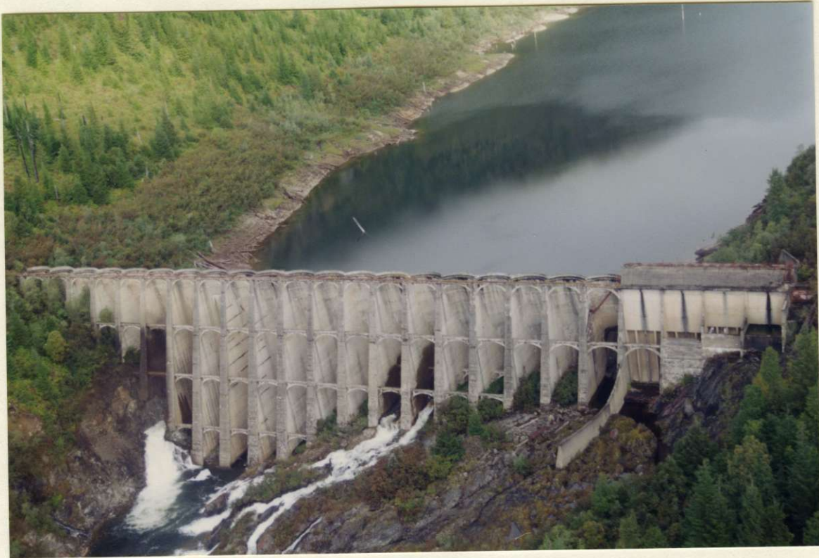
ANYOX CREEK HYDRO DAM HAS SEVERAL FAILED LOWER SECTIONS. A COST-BENEFIT ANALYSIS RECOMMENDS THAT THE SITE BE REFURBISHED.
