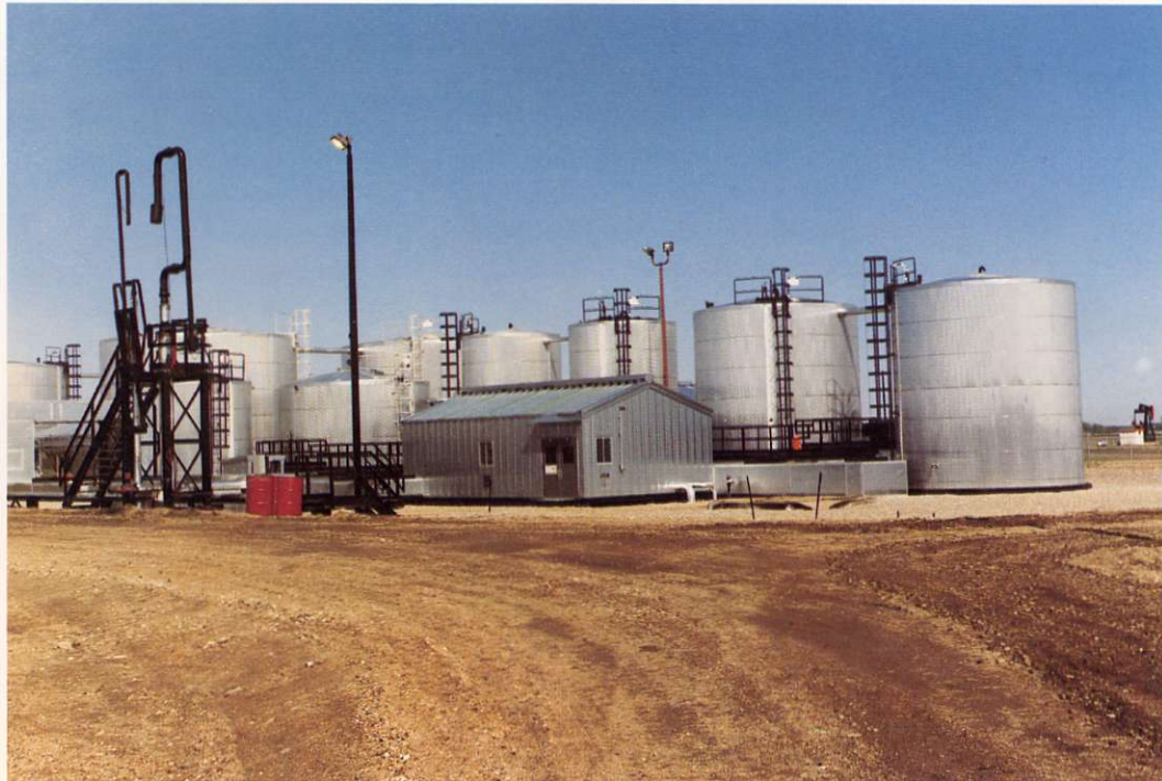
Westmin's new 3,000 bopd Elk Point cleaning plant is already operating above capacity.
