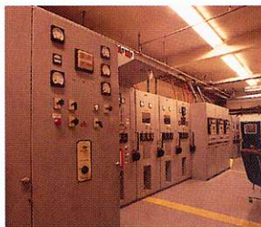
Power station control room.
