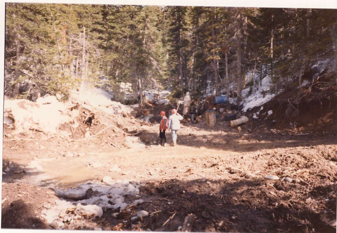
86-Roll 2-12 Coil stove and pump on Boulder Creek. Proposed portal location for adit by Canadian-United Minerals Ltd.
