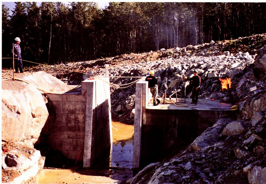
Effluent control structure at the Louvicourt tailings area, the first application of this technology in a mining operation
