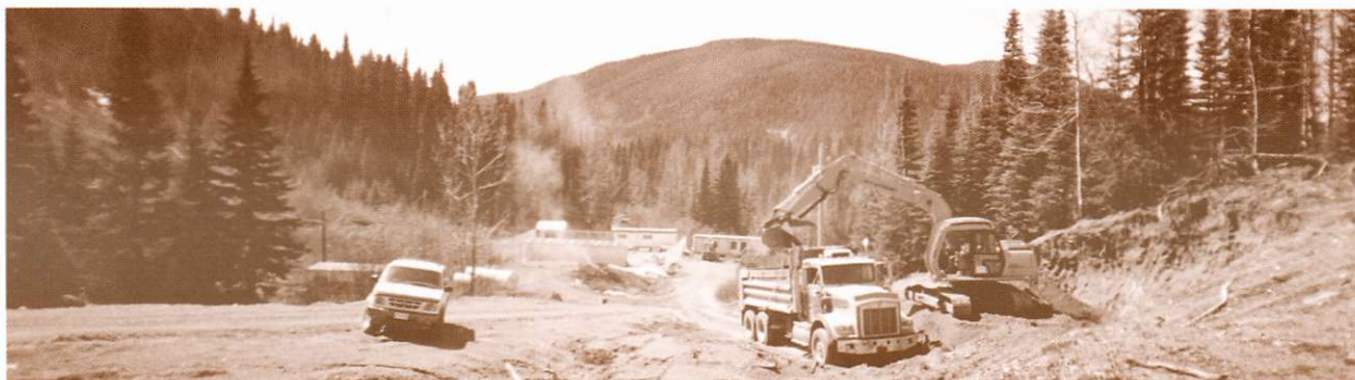
Pete Wright, Dale Pinkerton and Arnold Schmode adjusting the grade leading to the drill core compound.
