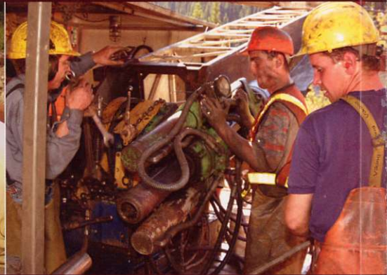
Diamond drilling from the portal in advance of the decline for the bulk sample program at the Bonanza Ledge Zone.
