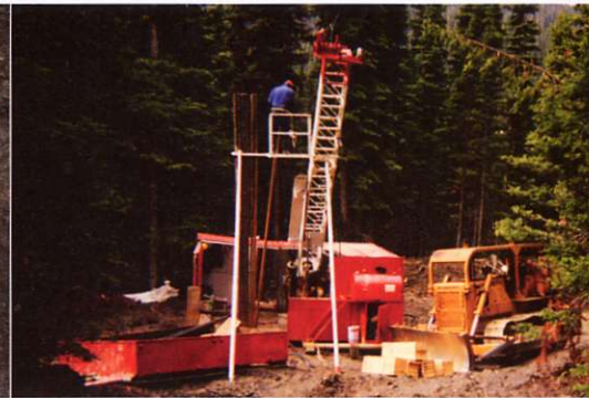
Setting up the drill rods on the Bonanza Ledge Zone prior to commencing the underground bulk sample.
