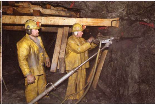
Changing the heading, drilling the next round to blast for the 10,000 tonne bulk sample to produce the first gold.
