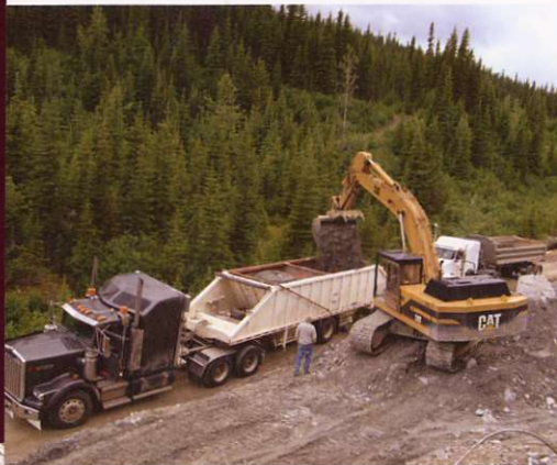
Loading mineralized material from Bonanza Ledge bulk sample for shipment to the Mount Polley Mill for processing.
