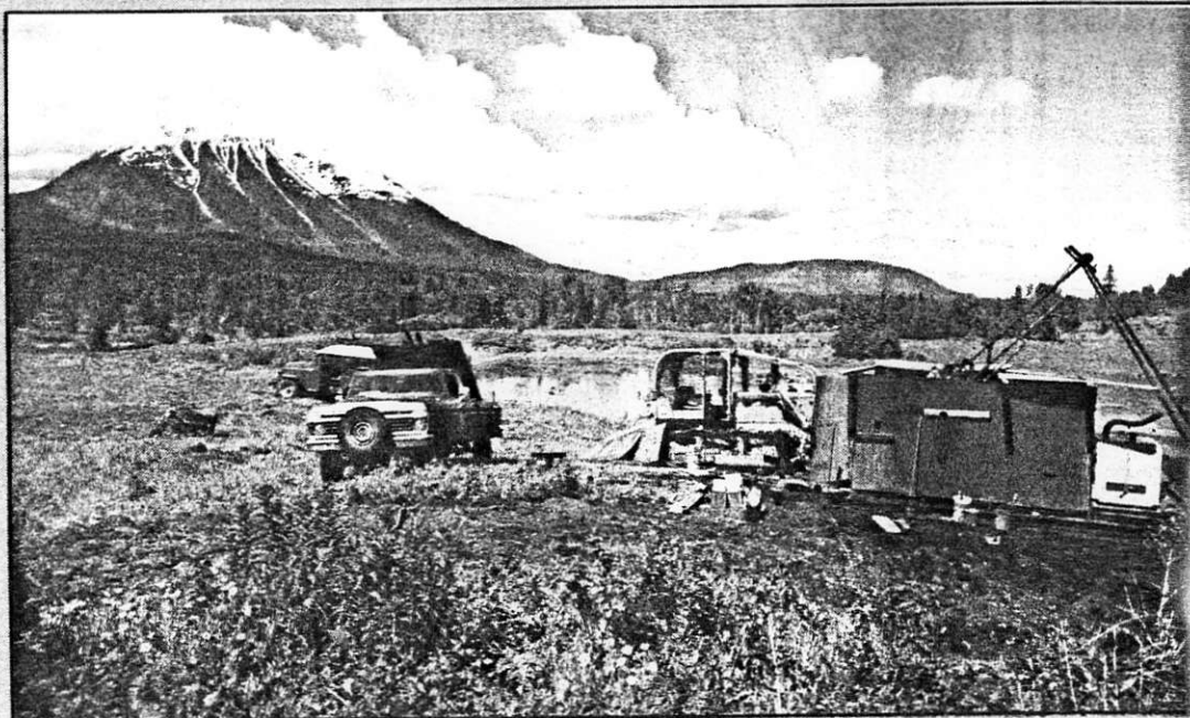
Diamond drilling to the south of the tailings pond at New Nadina's Silver Queen mine was conducted this summer to test the extension of the Chisolm breccia silver zone in the Owen Lake mining camp of west-central British Columbia. New Nadina has agreed to joint venture with Bulkley Silver Resources to develop the Owen Lake property.
