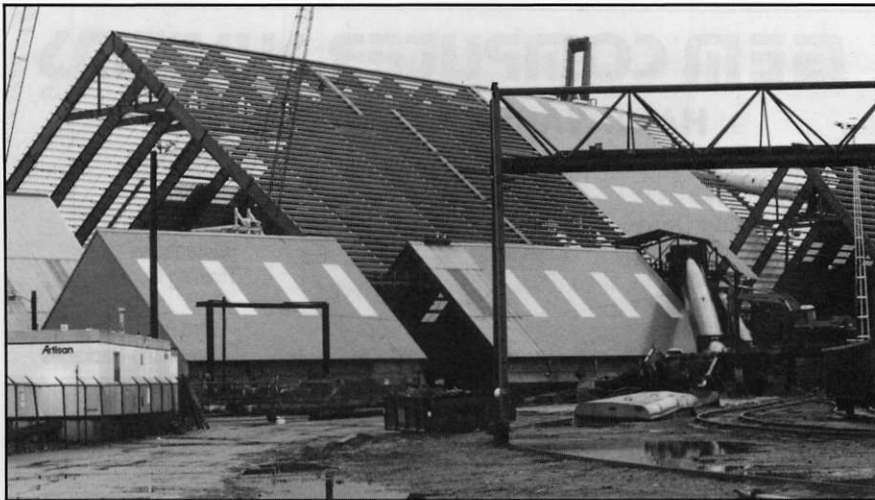
Vancouver Wharves just recently completed a $35-million expansion to handle lead and zinc concentrates from Cominco's Red Dog mine. The concentrates are then moved by rail to the company's massive Trail smelter. PHOTO: MARK BOWEN
