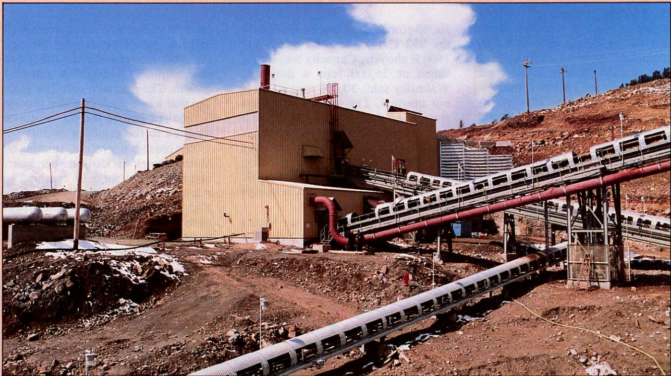
An extensive system of conveyor belts links Mascot's primary crushing plant to the mine's grinding mills.
