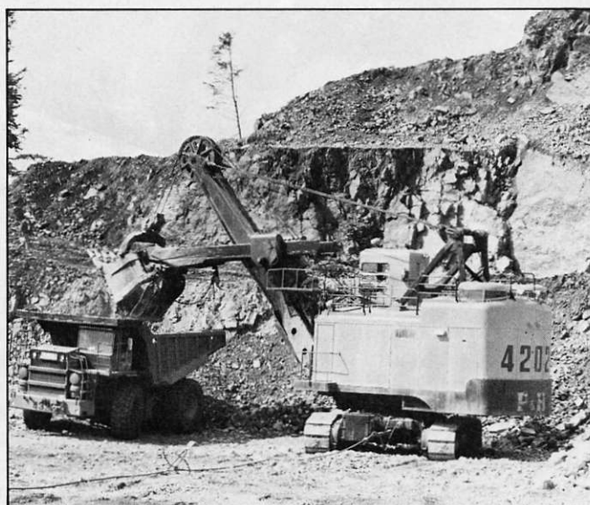
Mascot's open pit operation yields 2,700 tons of ore daily. Here, a P&H 1600 shovel loads one of the company's 60-ton Wabco haulers.
