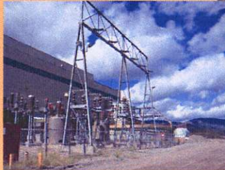
138 kv Power Supply
