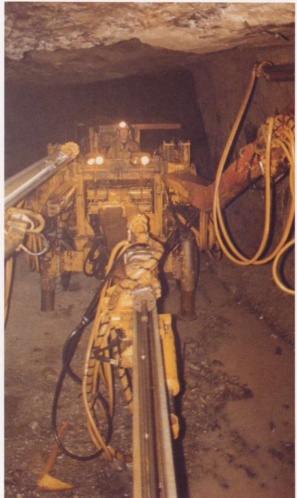
Twin boom drill jumbo, part of the trackless mining system employed at the mine.
