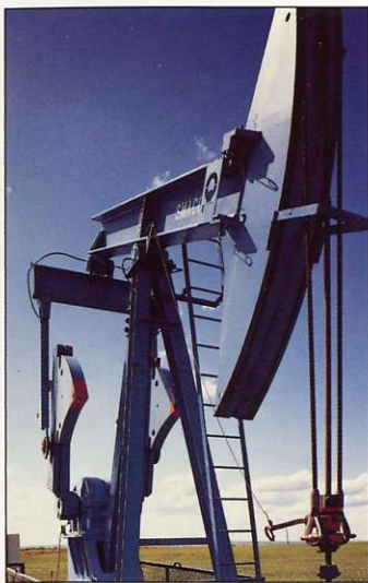
Pumping station, Steelman Oil Field, Saskatchewan.
