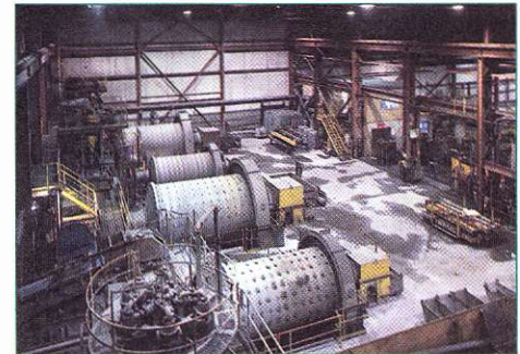
Grinding mills, Myra Falls Operations
