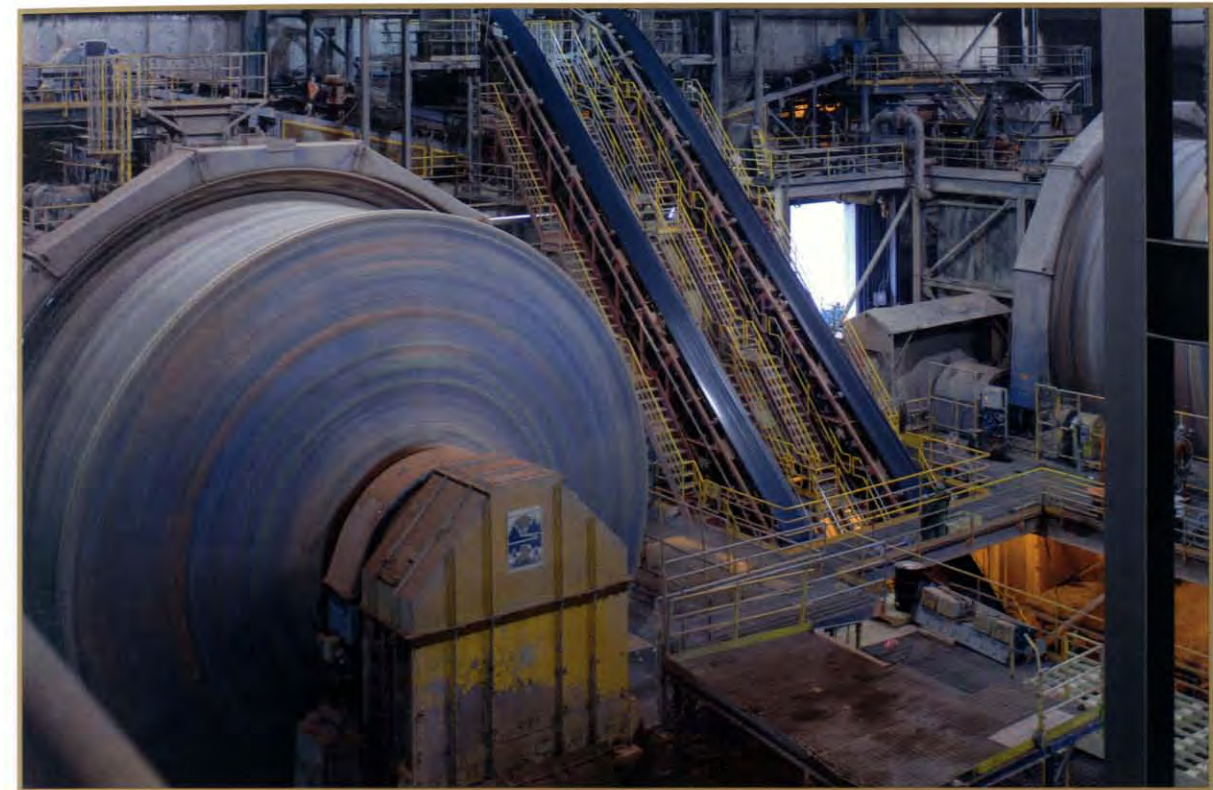
B- and A-Side SAG Mills, with conveyor from primary crusher in between, Kemess Mine
