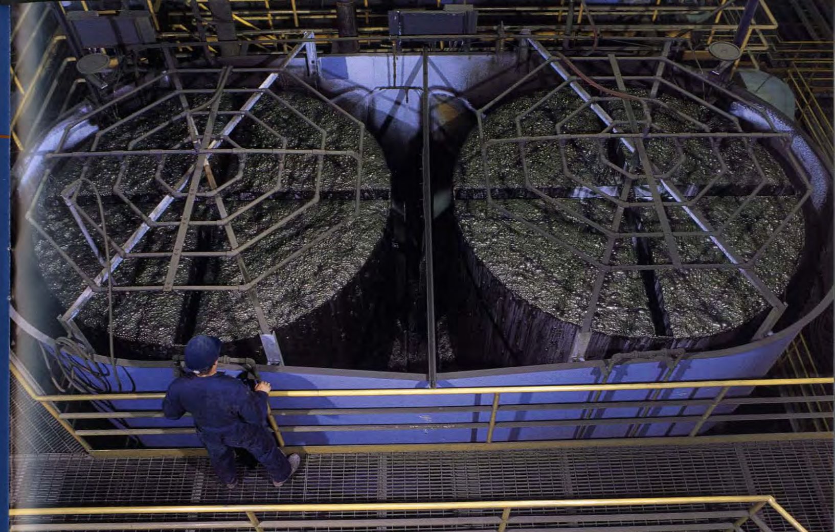
Column Flotation Cells – Gold and copper being recovered from the two new column flotation cells.
