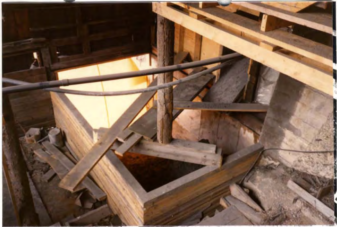
86-Roll 4 - 8 Ore concentrate is gravity-fed to a bin with an electrically heated cement floor. A similar bin is used for dry tailings.
