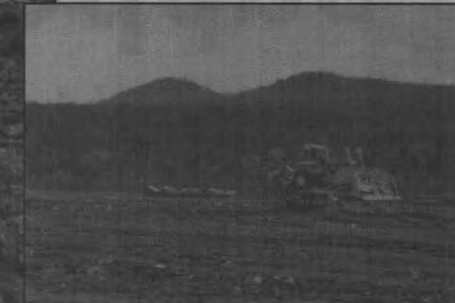
Dozer pulls a large log to level glacial tills and construct flat land.
