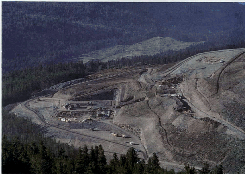
Aerial shot of Mascots Nickel Plate Mine. Cleared flat area upper right will be site of maintenance facilities. Central area will hold pebble and fine ore stockpiles. Grinding and aeration facilities are lower left, with cleared area in background for tailings.
