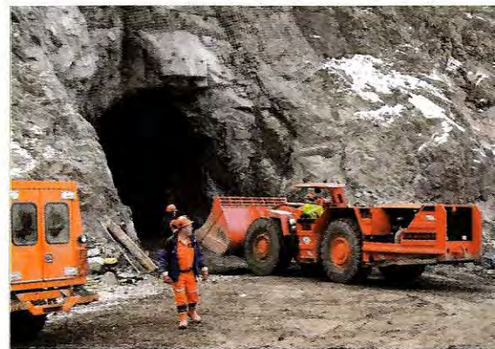
Richard Keane, shift supervisor from Procon Mining & Tunneling (left foreground) oversees continued work on an underground decline at the Afton copper-gold project in southeastern British Columbia. A 2-km decline is planned for the property, allowing drillers to complete 20,000 m of core from the underground workings, an effort designed to upgrade the measured and indicated resource to reserves.
