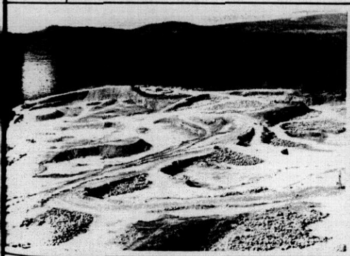
View from top of quarry toward quarry shop — mid-upper part of picture. Riprap boulders stockpiled for future use.
