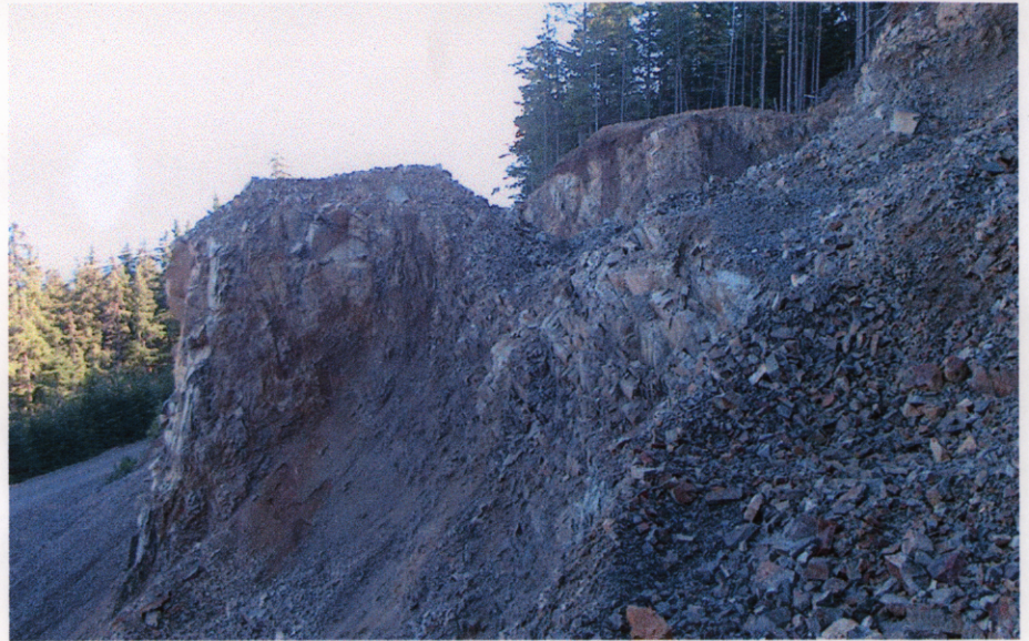
October 3, 2001 - Dude Claims on Texada Island - former Tex showing MINFILE 092F276 - Re-excavated roadcut
