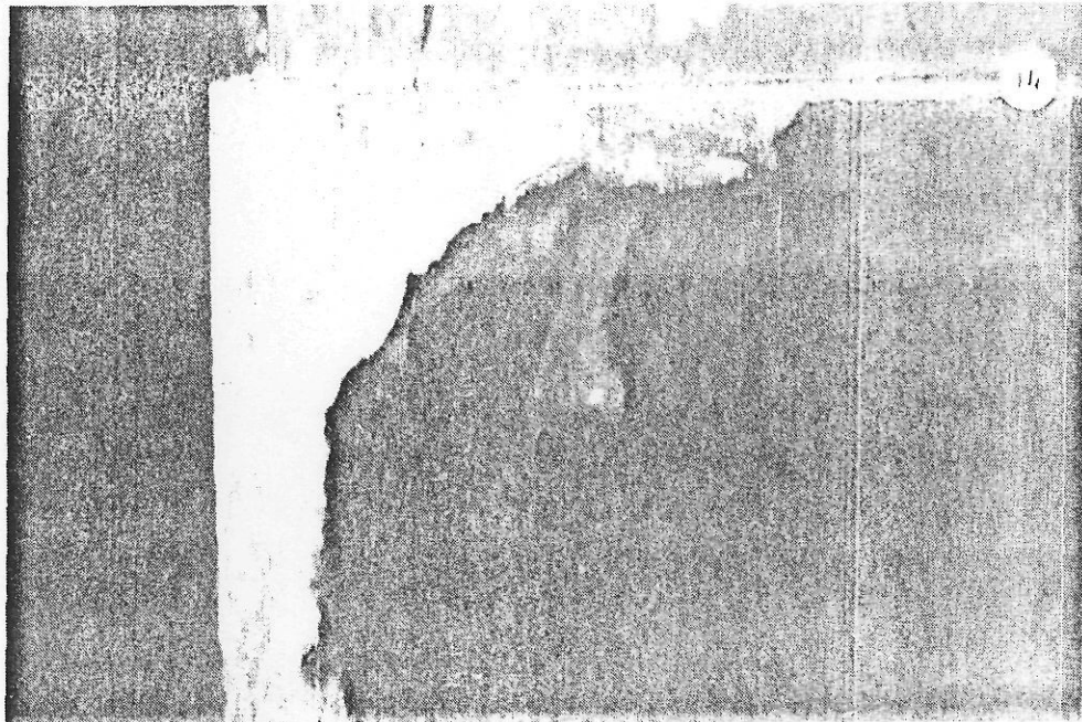
Figure 14. Corroded Steel Support.
