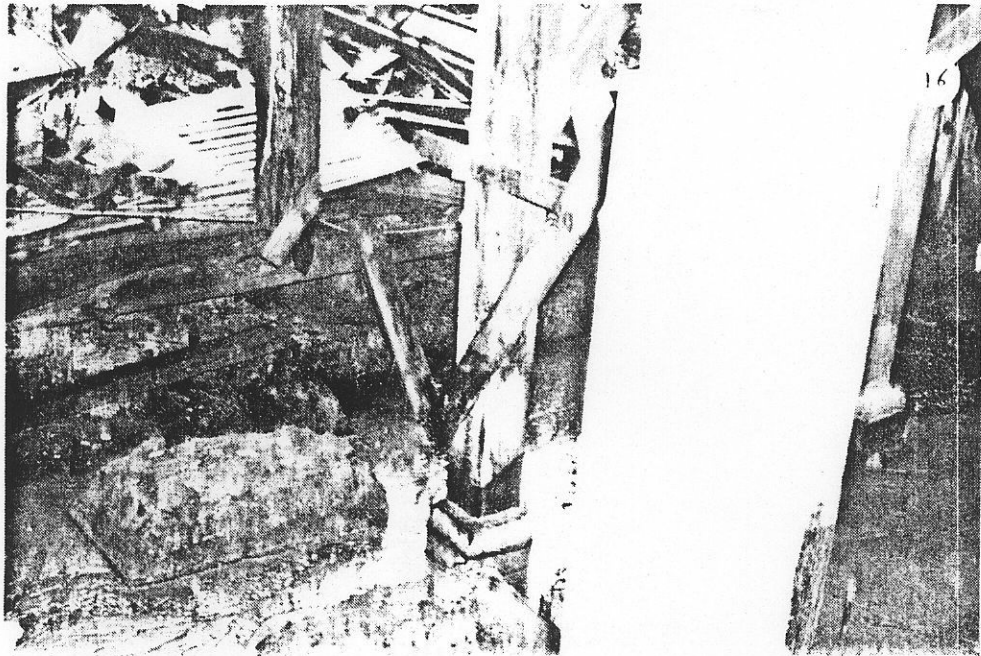
Figure 16. Timber Elements in Relatively Good Condition.
