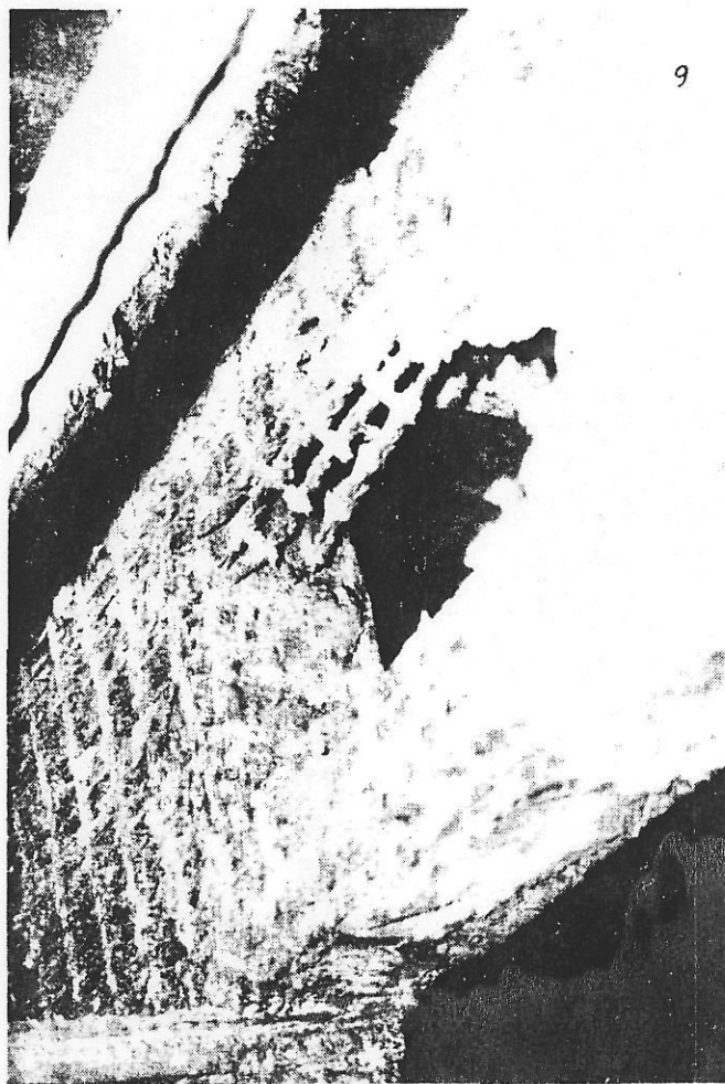
Figure 9. Badly Corrode Concrete Beam.
