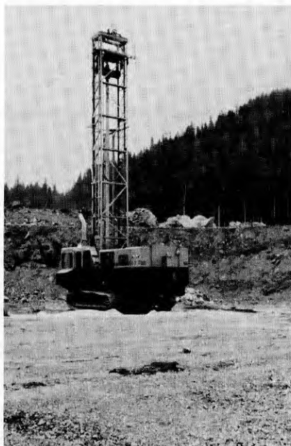
Nine-inch holes are drilled in the open-pit by mobile rotary Diesel-powered rigs.
