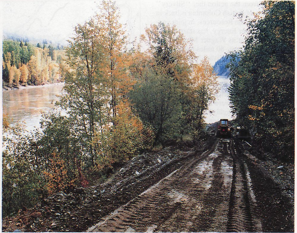
Front end loader on roadway to mine portal. The Fraser River can be seen through the trees.
