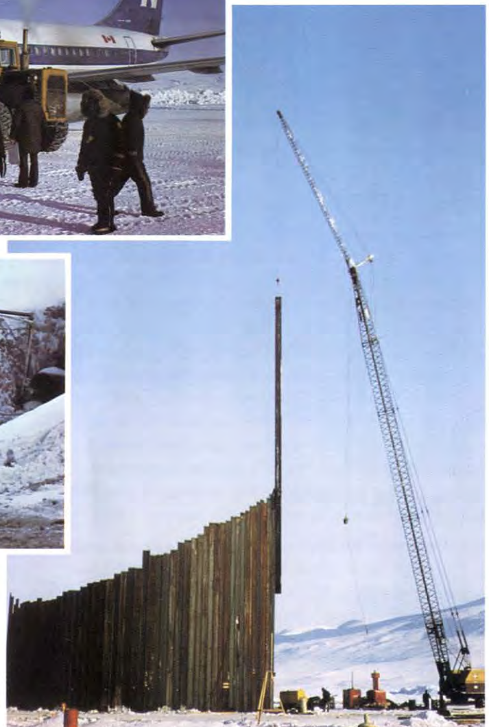
Threading of 80 foot long linked sheet piles through ice of Strathcona Sound to form one of three 70 foot diameter cells in dock construction.
