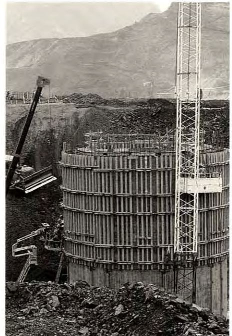
New truck dump structure rises from the ground during construction; most of the structure was subsequently buried.
