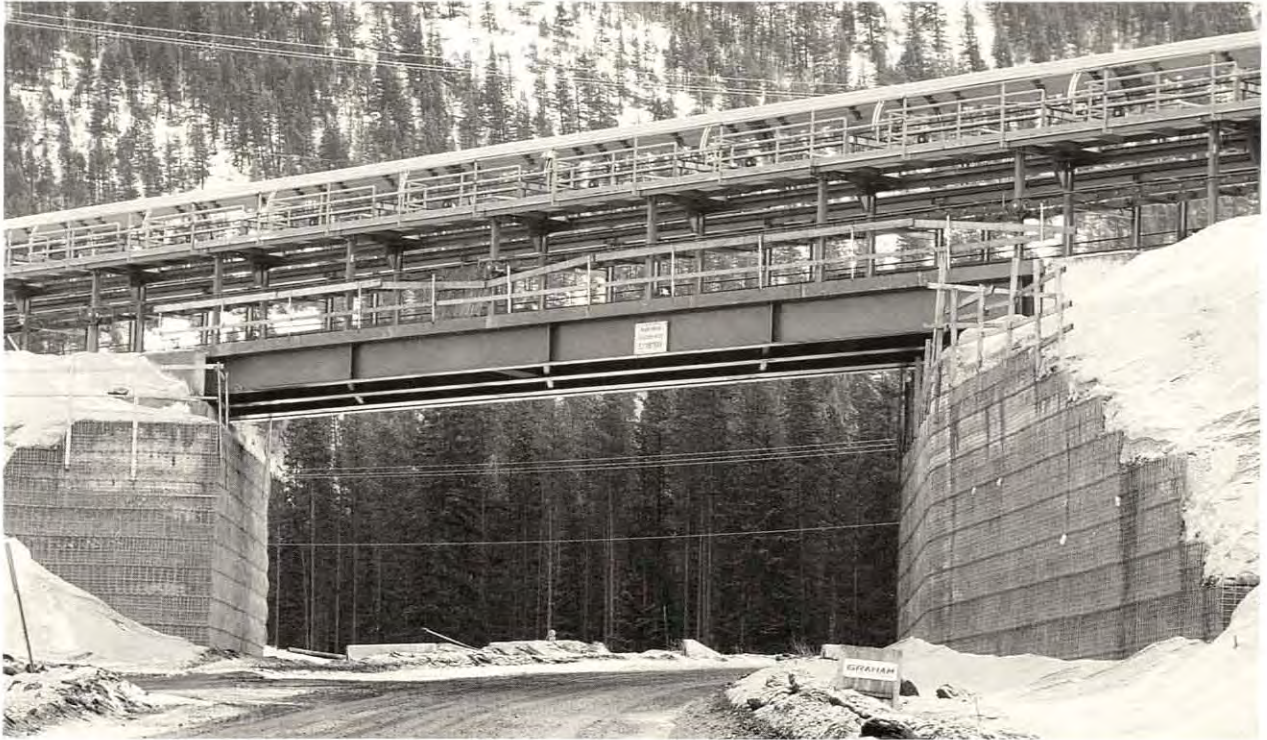
Overview crossing of mine access road providing view of interesting design and construction challenges
