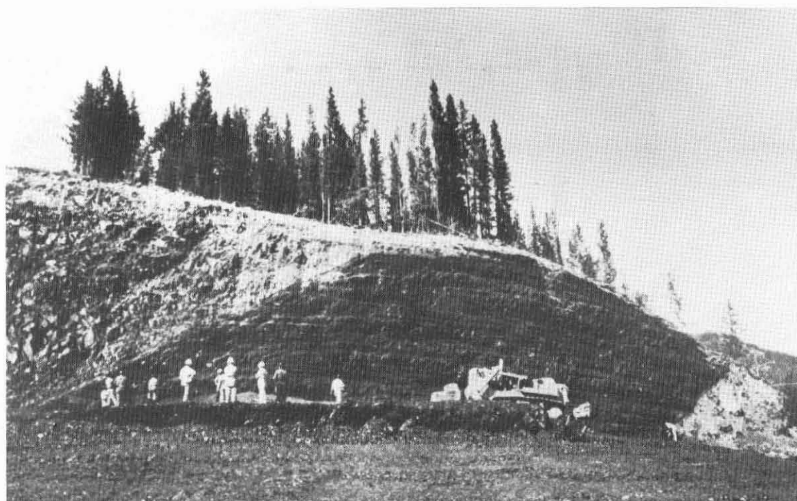
An early experimental excavation at Kaiser's Elkview operations shows typically sloping nature of the deposit.
