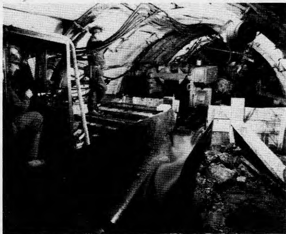
In underground mining, Kaiser Resources uses the hydraulic method, applying water under high pressure to dislodge coal from the seam and fluming the coal out of the mine in slurry form. The hydraulic monitor is operated from a module 40 feet from the face, a major safety feature.
