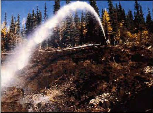
Hydraulic ground sluicing uses high pressure water jets for a low cost removal of thawed organic cover from the pay gravels.
