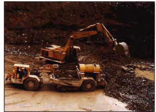
In the 1986 bulk sample at Moyie River, B.C., a hoe-scraper operation excavates a 40 foot deep pit to expose the bedrock pay channel.
